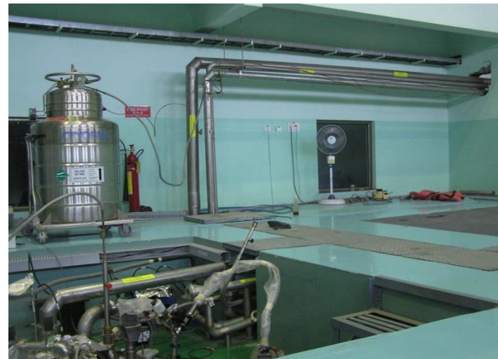
Cryogenic Transfer lines for VTS
